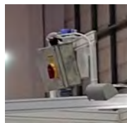
Mains Power Box & Cable Mounted Above Stand
